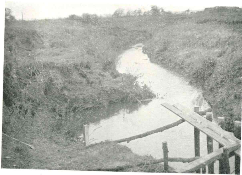
Rye Internal Drainage District. River Seven. Eroded bank.
