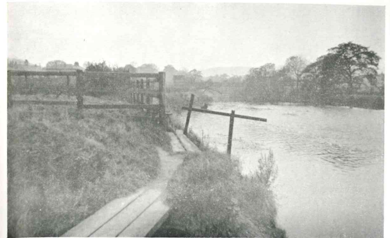
River Aire. Bingley. Erosion of footpath.
