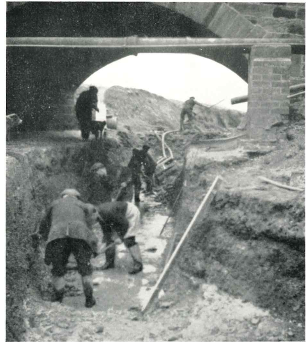
Dearne & Dove Internal Drainage District. Bulling Dyke. Trench for Culvert under Broomhill Bridge.
