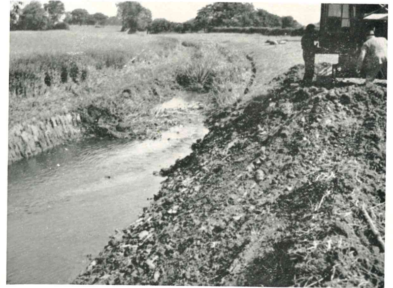
Foss Internal Drainage District. River Foss. Work in progress above Towthorpe Bridge.
