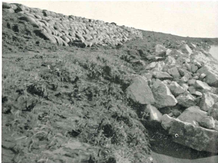
Breach temporarily repaired.
