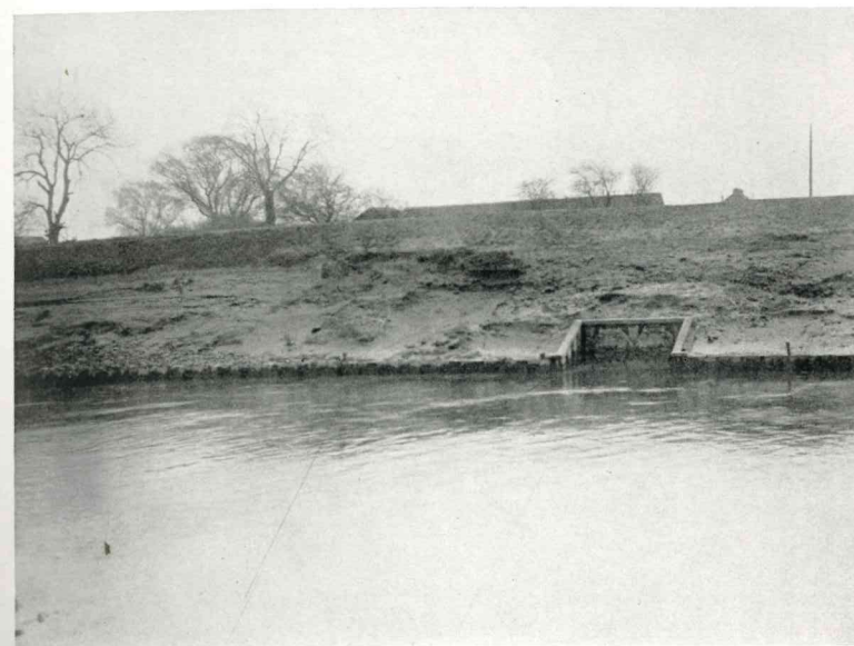
Dutch River. Swang Clough. Erosion of bank behind piling.
